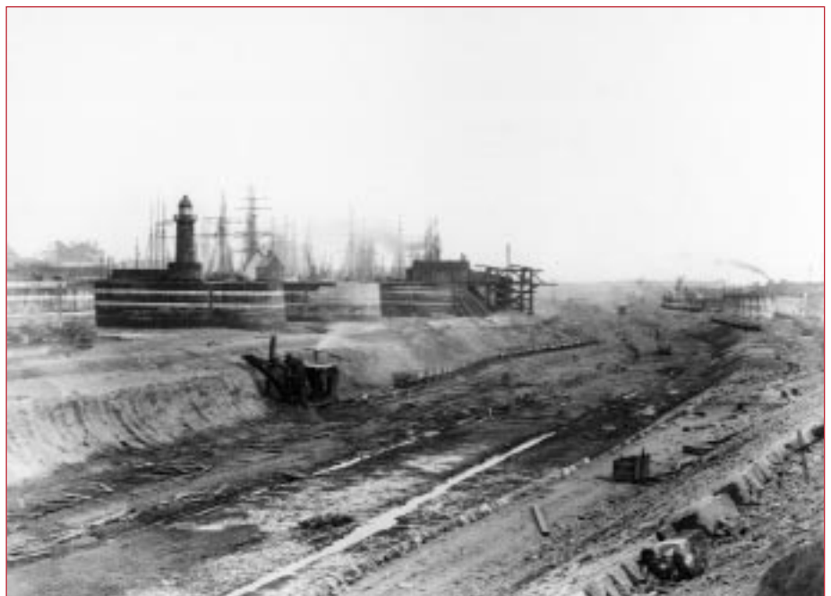
Excavating the Manchester Ship Canal at Weston Point, Cheshire c.1888, taken from one of the Manchester Ship Canal Company's original glass plate negatives. Manchester Ship Canal/The Boat Museum Trust.
